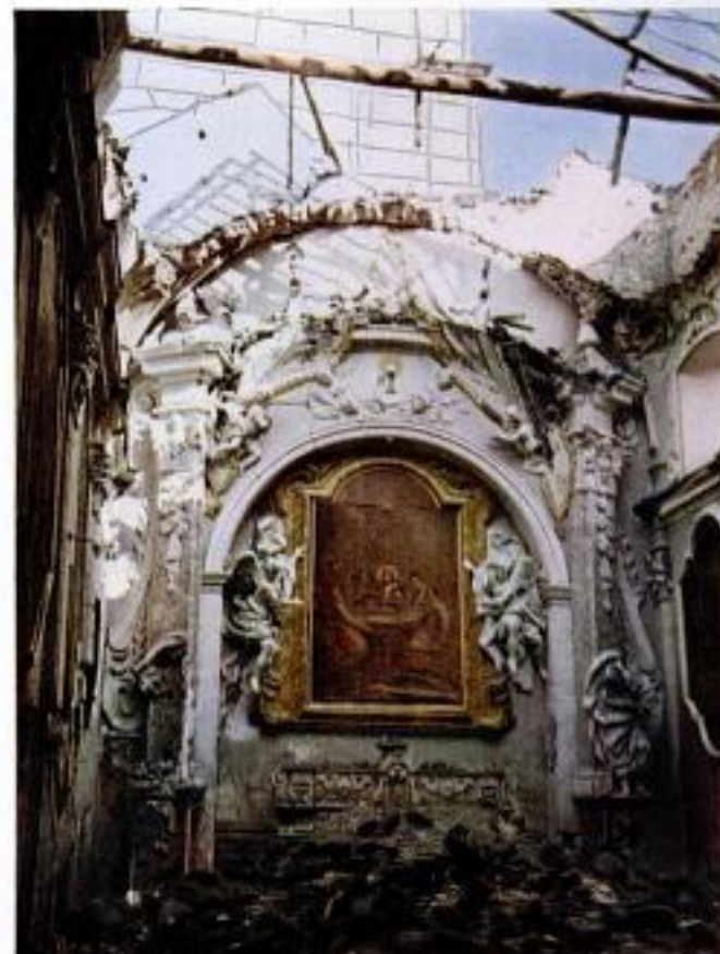
CAPUA CATHEDRAL CHAPEL, with painting of Last Supper, baroque sculptures, was damaged. In the background, through gaping roof, Ninth Century bell tower is visible.
